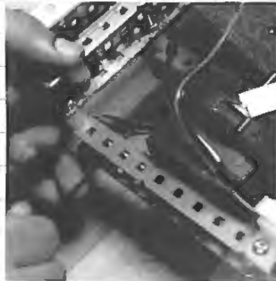
Tightening Base Motors
